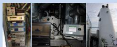
Figure 2: Experimental setup with measurement equipment and chimney
